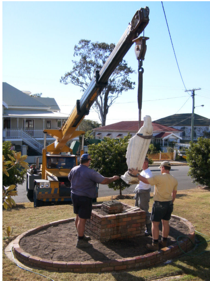
Workmen install the statue of our lady in the front of the property in Walnut Street Wynnum
